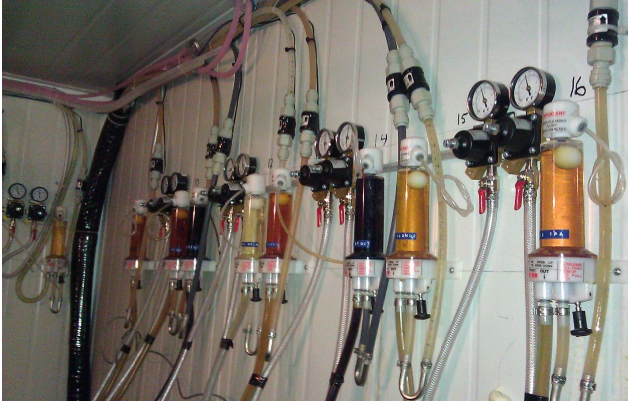
Figure 4: flow meters in cooler
