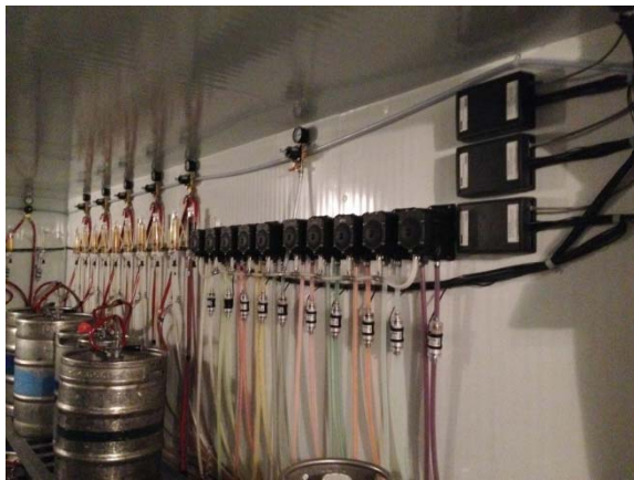
Figure 6: flow meters with beer pumps
